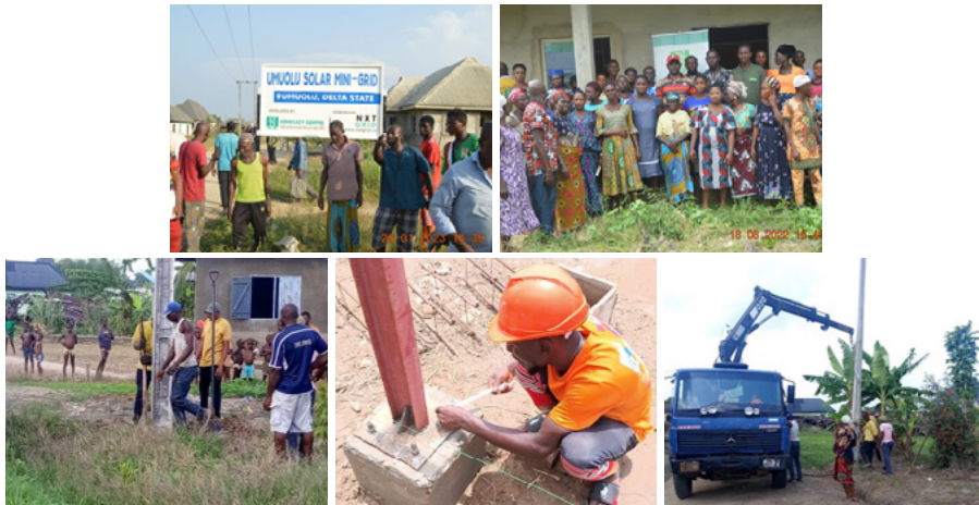
Figure 6.7: Local communities in the Niger Delta and local solar mini-grid installations. 143
